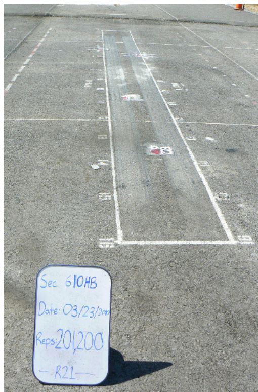
Figure A.24 610HB - PG 64-28 PM - 64 mm: Section photograph at test completion.
